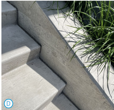
D Concrete Steps
